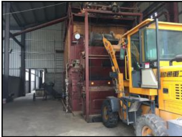
10t/h 蒸汽锅炉
